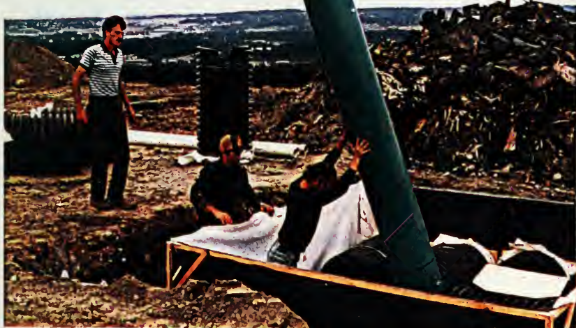
A11: POSITIONING MONITORING WELL. INSTALLATION-READY 1.5m LONG BIG "O" TILE SHOWN IN BACKGROUND.
